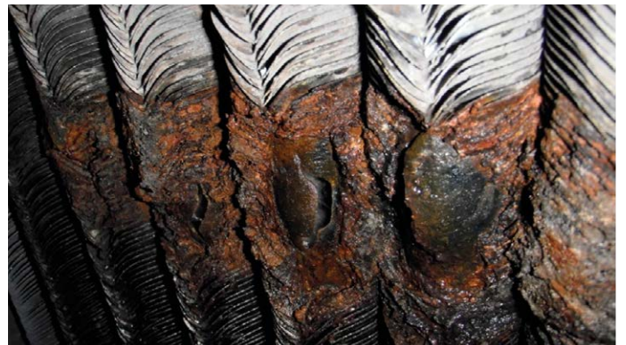
Severe acute corrosion of ACC tubes can totally paralyze a power plant
