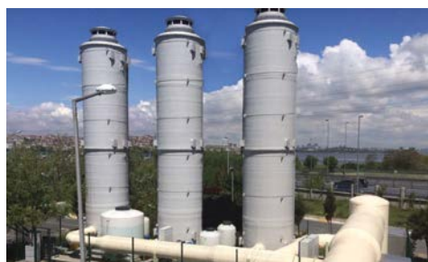
Biotricklingfilter remove odorants of waste water treatment plant
