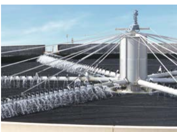
Biological water treatment
