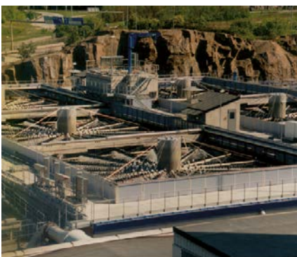
Nitrification Filters, Gothenburg, Sweden
